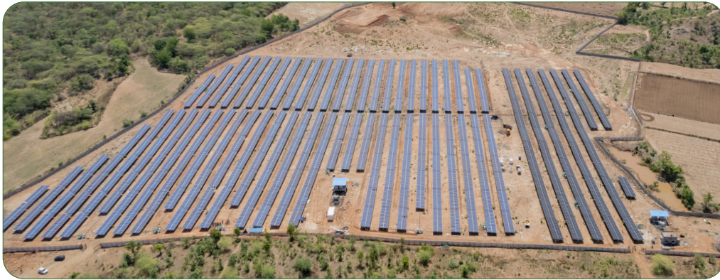
1 MW solar power plant has been installed to reduce carbon emissions and set a benchmark
