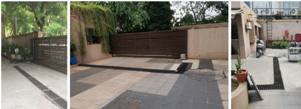
Three 120 m 3 percolation wells collect 100% of rainwater from all areas to recharge the groundwater table
